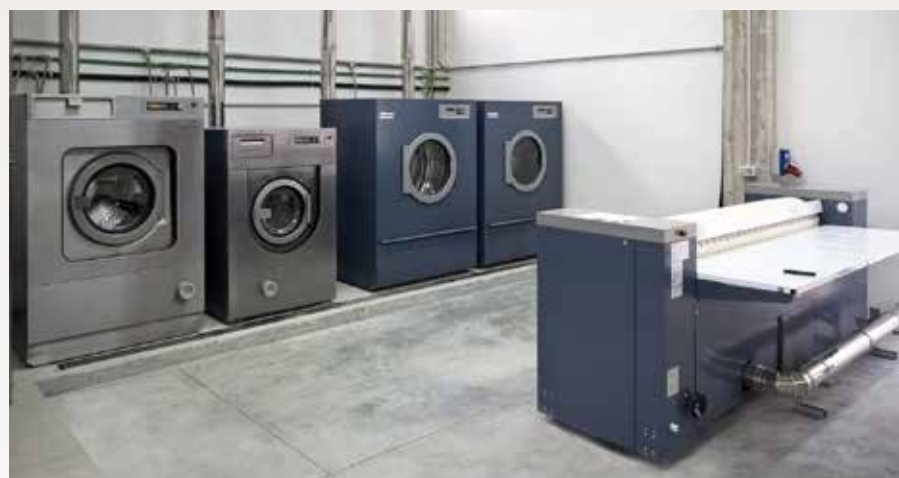
Double the facilities: The laundry service for the region's accommodation establishments is combined with a classic laundrette for locals and guests.
